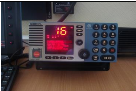
VHF radio station
